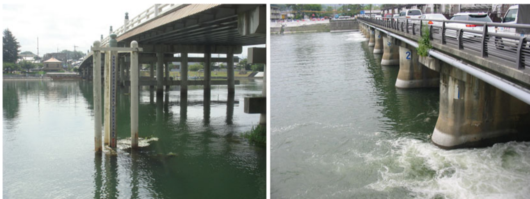
Fig. 10 Torii River Gauging Station and Seta River Weir.
