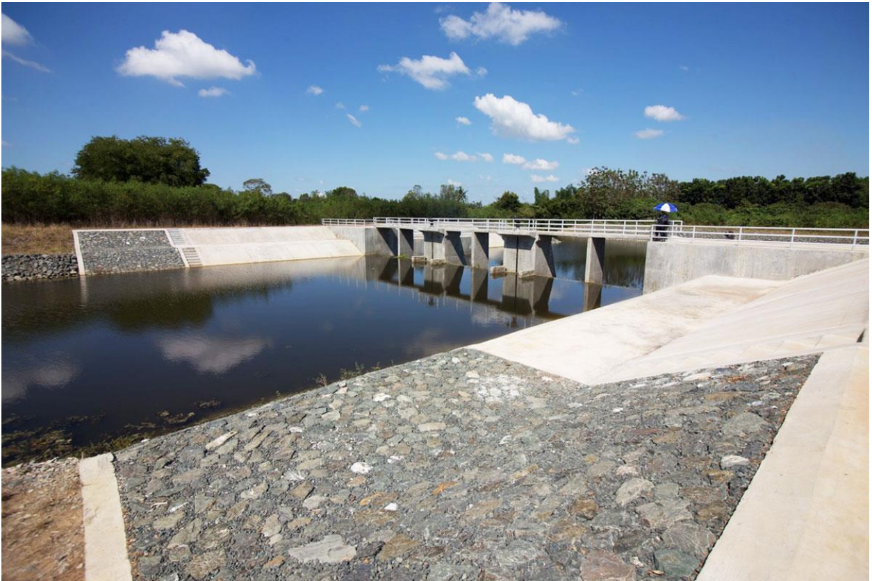
Photo: Weir at Khao Daeng Pattana Village. (Source: salika.co)
