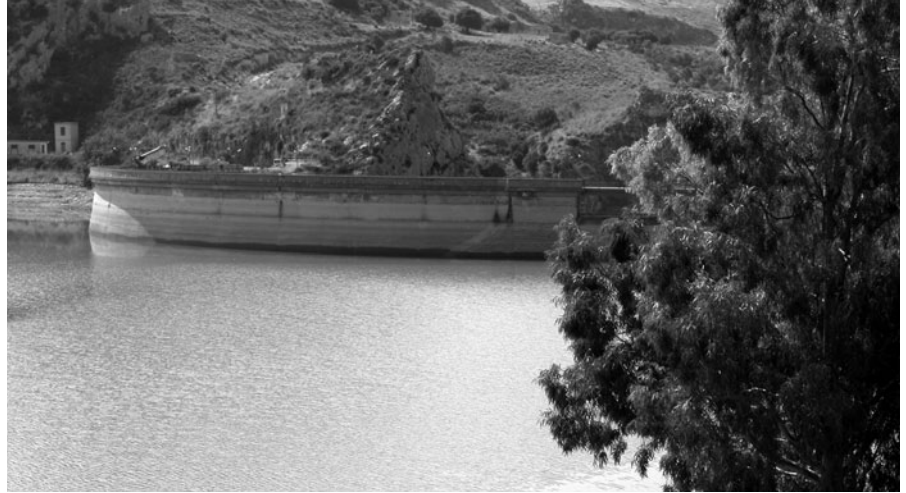
Lake Arancio dam. On the dam's wall the signs left by the water at different levels are easily visible.
