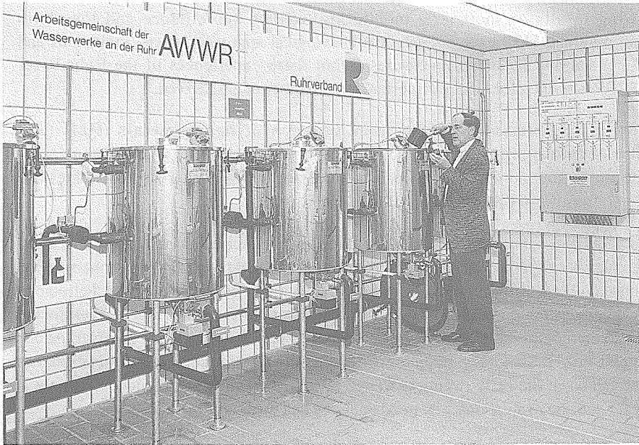
Fig. 8.3 Monitoring and sampling station at Fröndenberg
